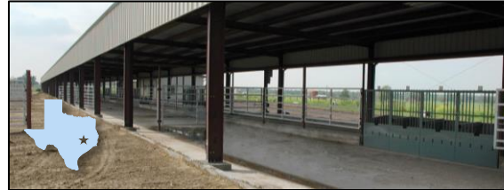
The largest individual feed intake system in the southern United States.
